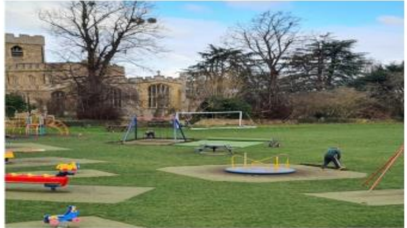
New surfaces for the play equipment go down at the recreation ground.
