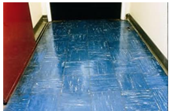
Asbestos containing floor tiles in a corridor
