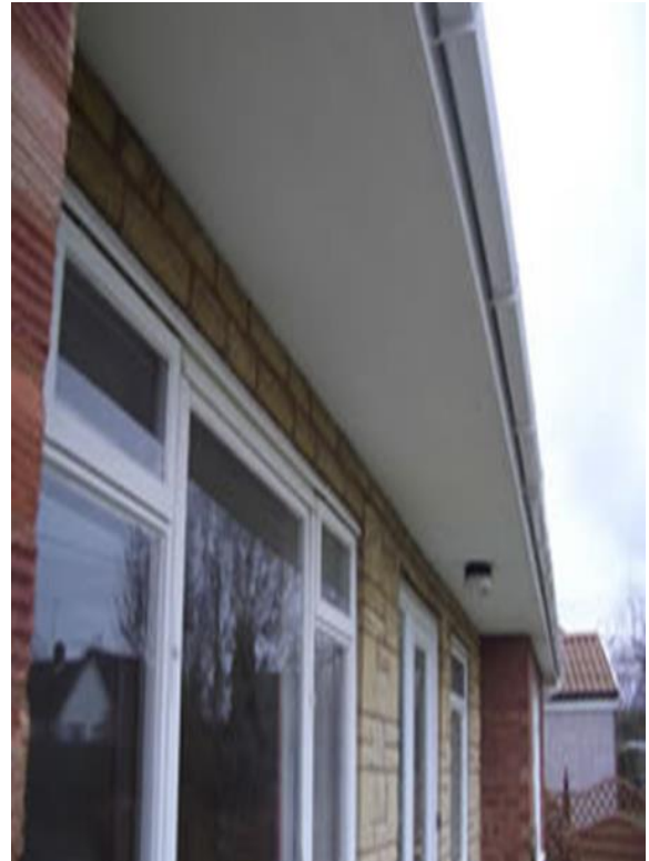
Pieces of Asbestos Insulating Board (AIB)
