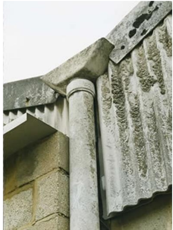
Asbestos cement downpipe, hopper and profile sheet
