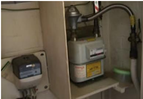
Asbestos panelling around a gas meter
